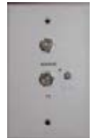
Antenna Power Supply
