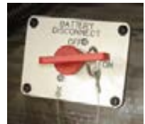
Battery Disconnect Switches
